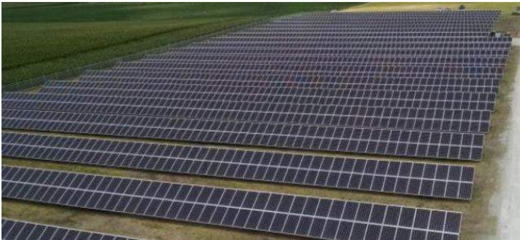
Example Photovoltaic Array
