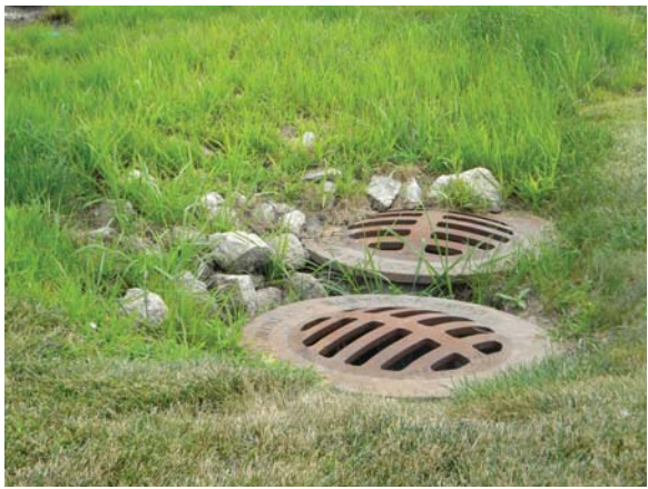
Drain inlet, mowing obstruction
