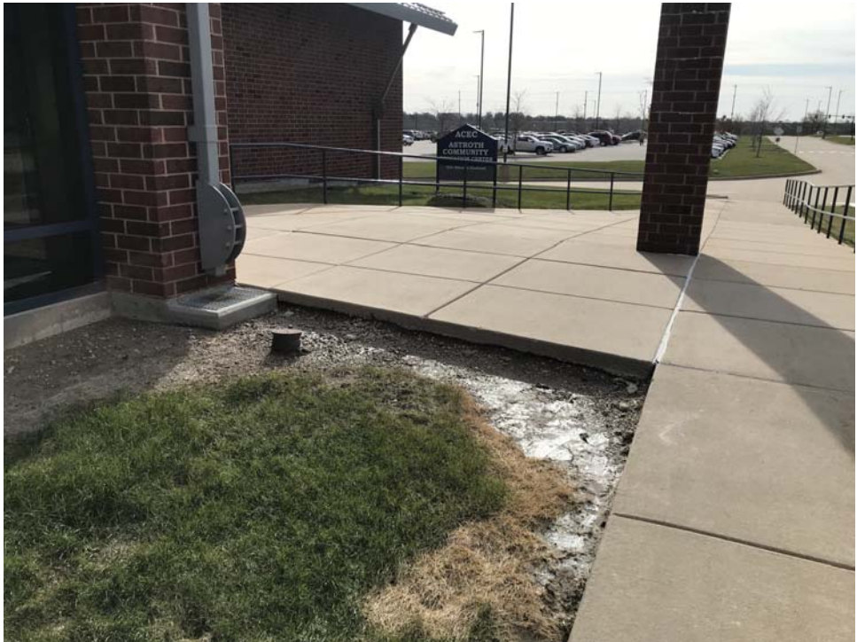
Typical condition at building entrances
