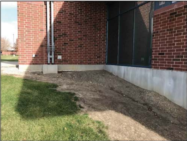
Erosion along west side of Fitness & Recreation Center
