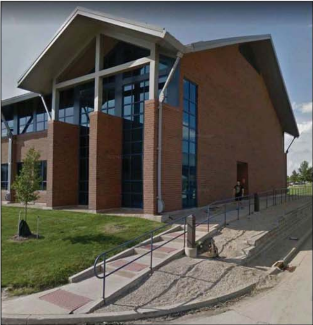
Gravel displacement and erosion at the southeast corner of Instructional Commons Building (east)
