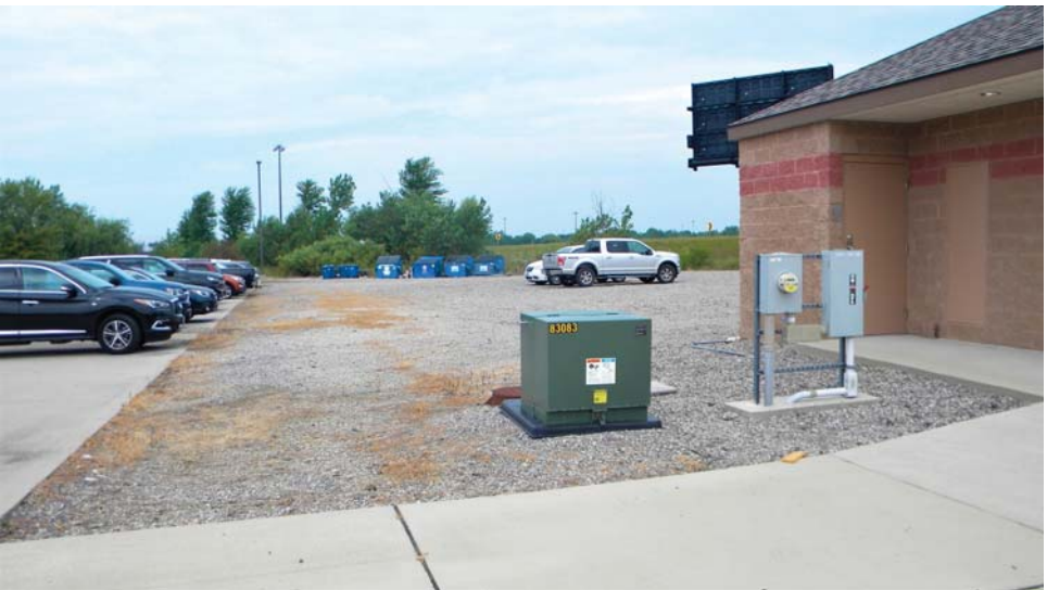
Exposed utility equipment
